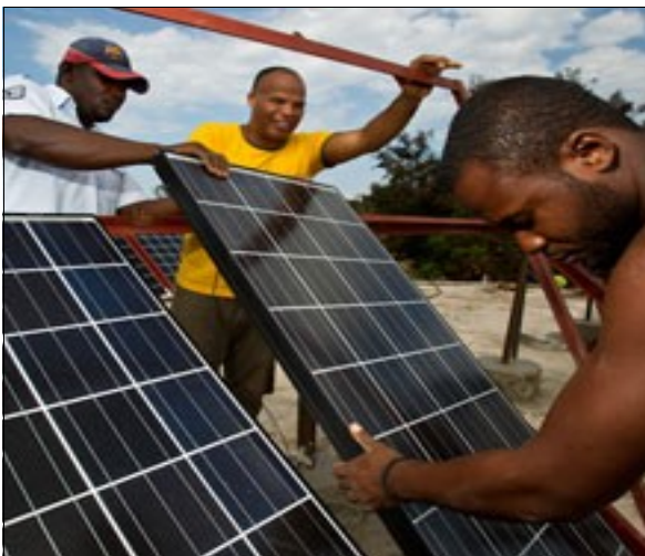
Rotarian Christopher Castor (middle) and Haitian volunteers install solar panels to run a medical clinic and water well for a village on the island of La Gonave, Haiti.
